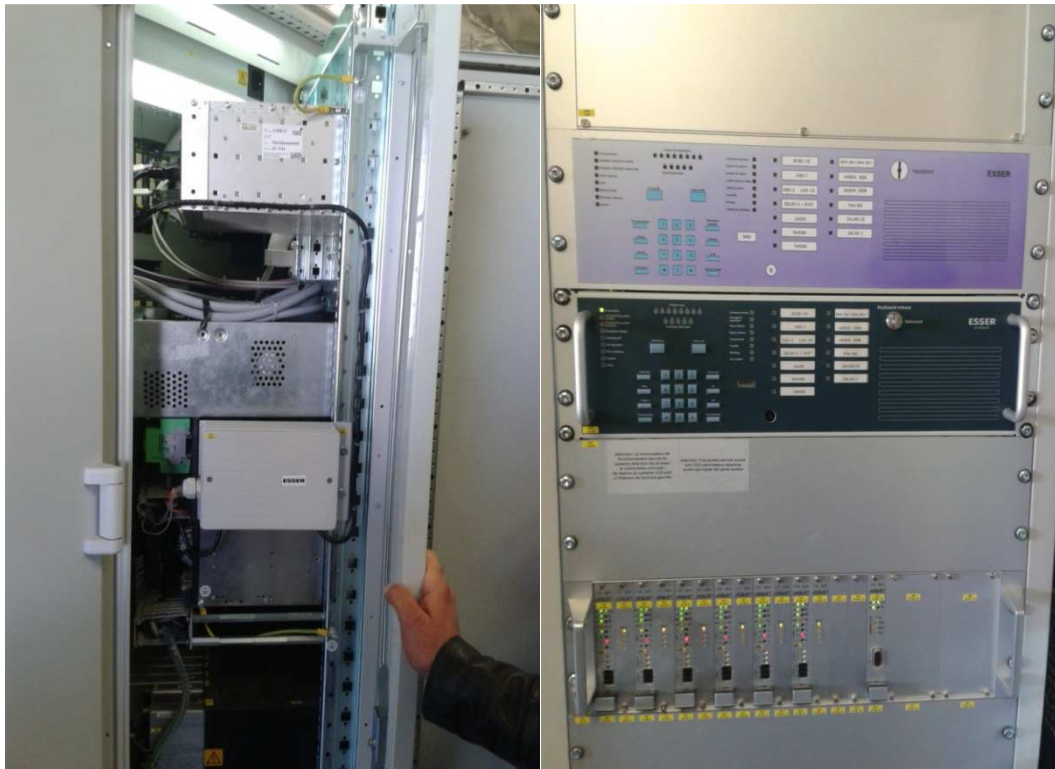
Figure II.15 : armoire de commande Honeywell.
