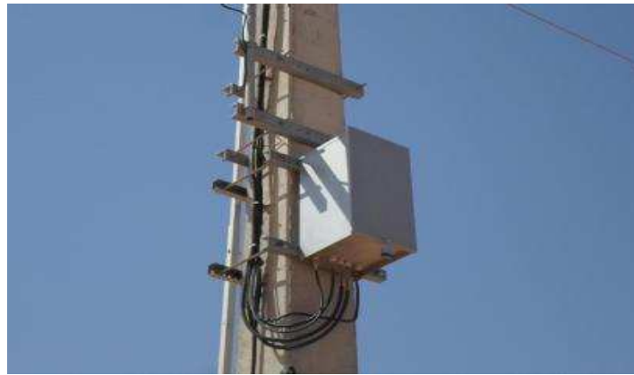
Figure III.5 Le coffret sur terrain
