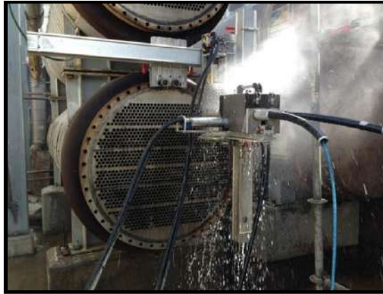
Figure 4 Automated equipments exchanger cleaning [1]
