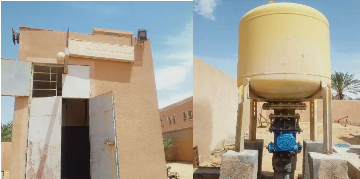
Figure II.7 : Station de pompage
