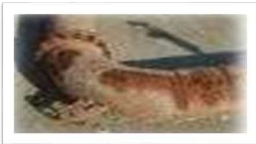
Figure I.1 : la corrosion uniforme
