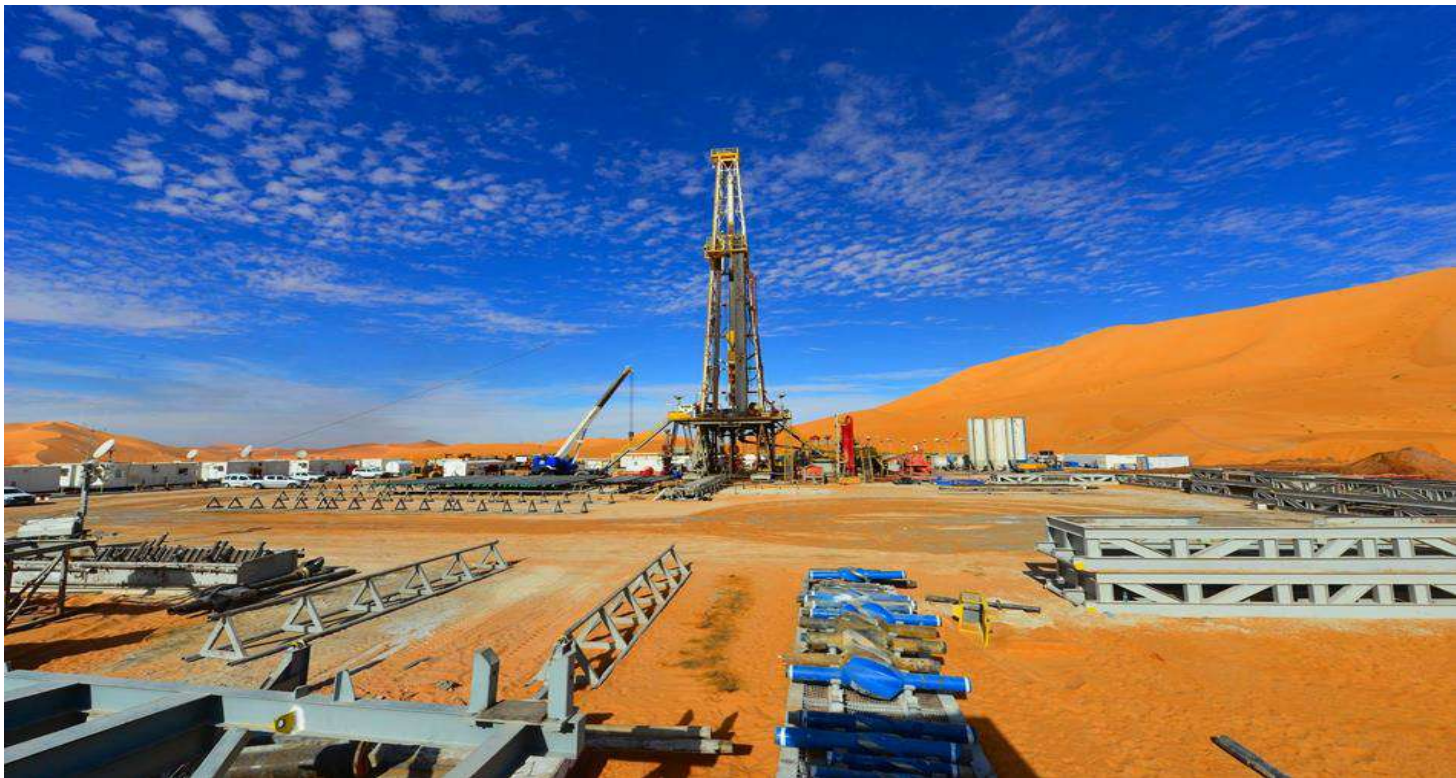
Figure I.1. Plateforme pétrolière Onshore[2]
