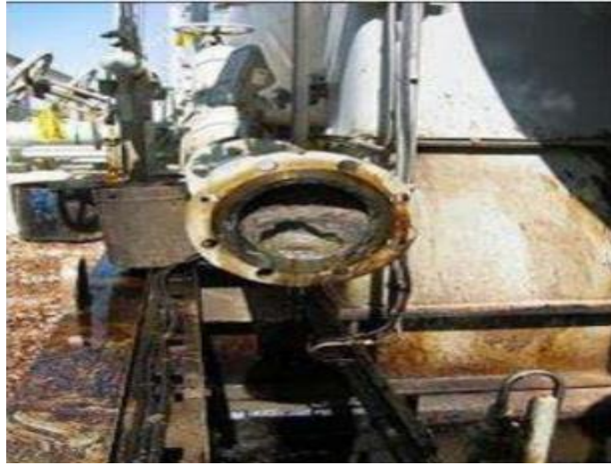
Figure IV.25: blockages of flow lines.
