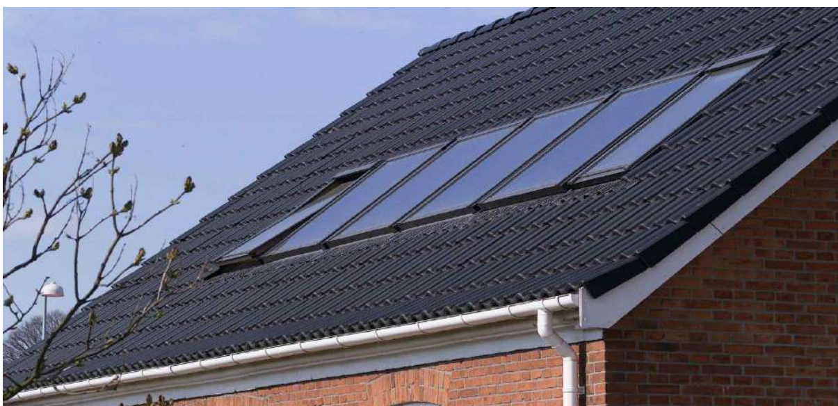
Figure (I.8) Roof installation of air heaters ( solarheateurope.eu )
