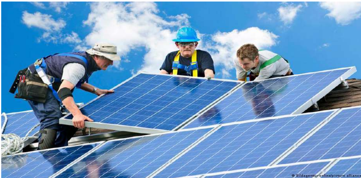
Figure (I.3) Photovoltaic panels (Gero Rueter, 2021)
