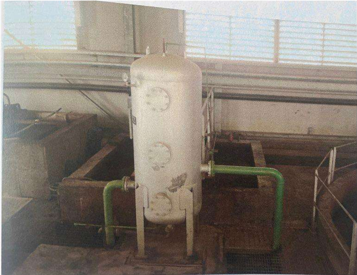
Figure 5: La cuve de floculation : S-103
