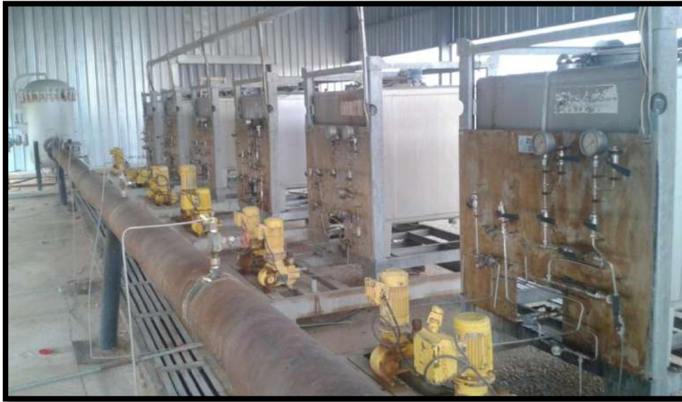
Figure (14): Station de traitement [17]
