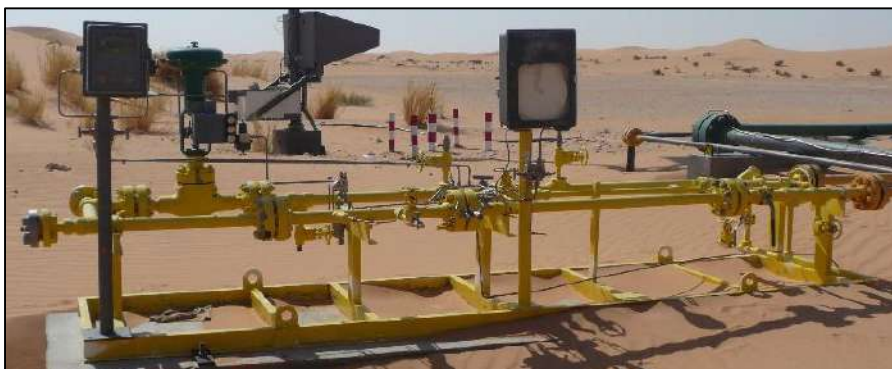
Figure I.6: Skid de Gaz lift
