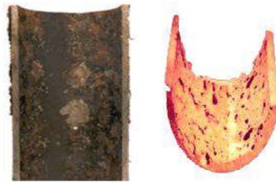
Figure I.5: Effet De Corrosion
