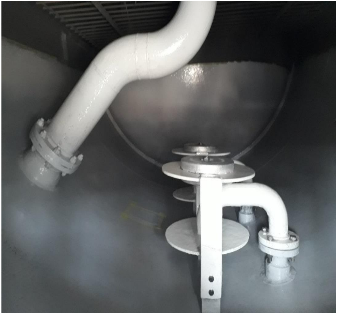
Fig .III.13: the internal surface of desalter after applied the recommendation above [26]
