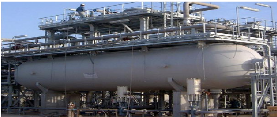
Figure I- 5: HP V.101 separator[02]
