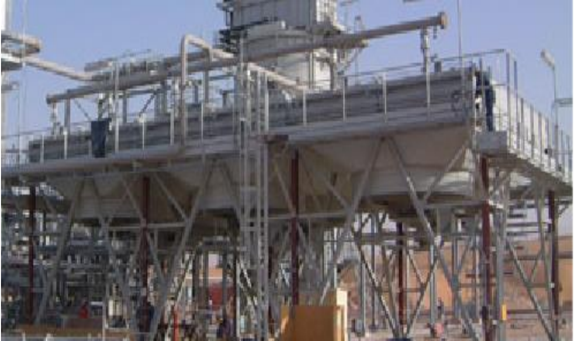
Figure I-9 :crude cooler (Air coolers) E.101[02]
