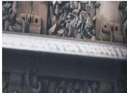
Figure I.39: Rail Head Corrugation
