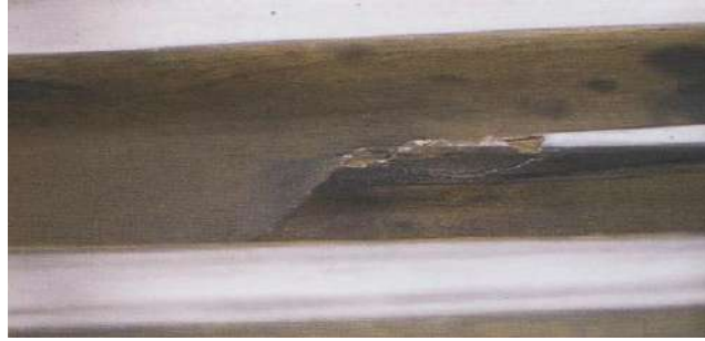
Figure I.43. Damage crossing nose
