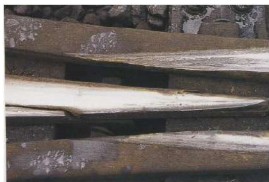
Figure I.36: Point and Splice Rails Separating
