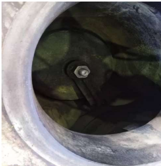
Figure (3-4): Check valve failure discovery.
