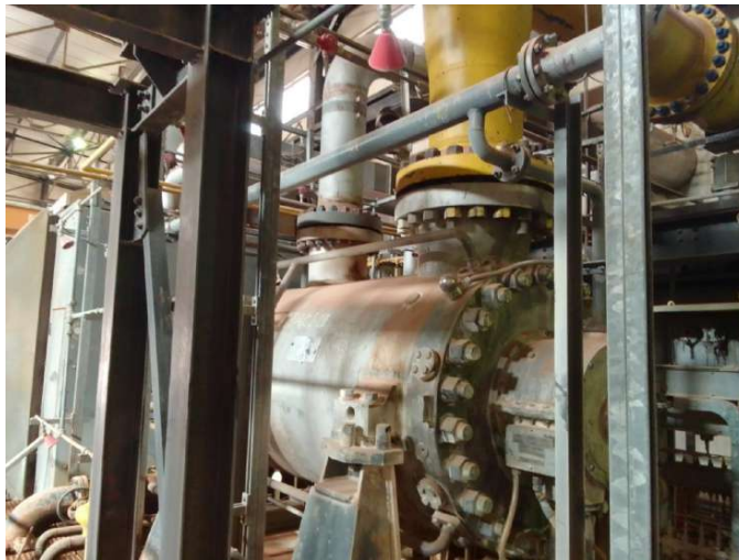
Figure (1-4): a compressor using in LPG 2 unit at SIC.
