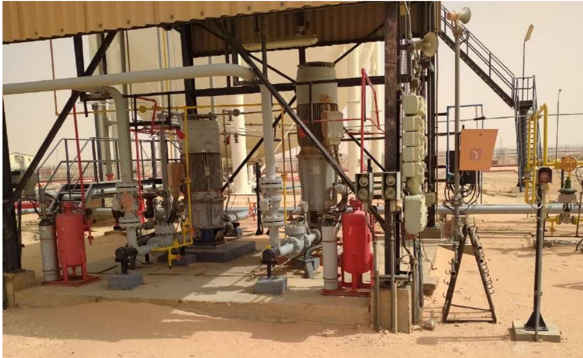
Figure 25 LPG pumps (P 703A-B)
