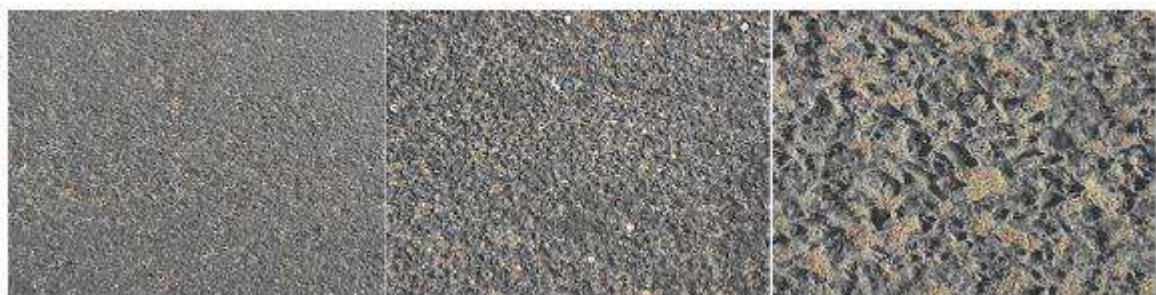
Figure (II.14) pavement in the time "corrosiveness"
