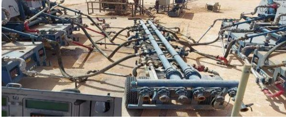
Figure I. 22: Hi/Lo Pressure manifold [22]
