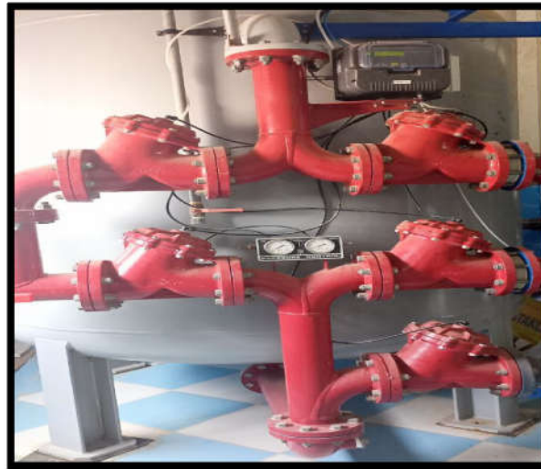
Figure III.12: Ensemble des vannes hydrauliques.
