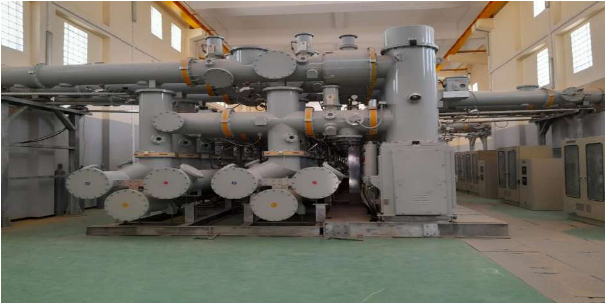
Figure III.4. Poste blindé de tension 400 kV
