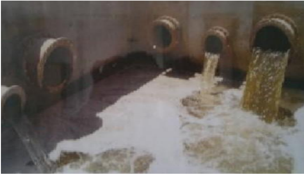
Fig (III. 5): Wastewater inlet to the station (degassing basin).
