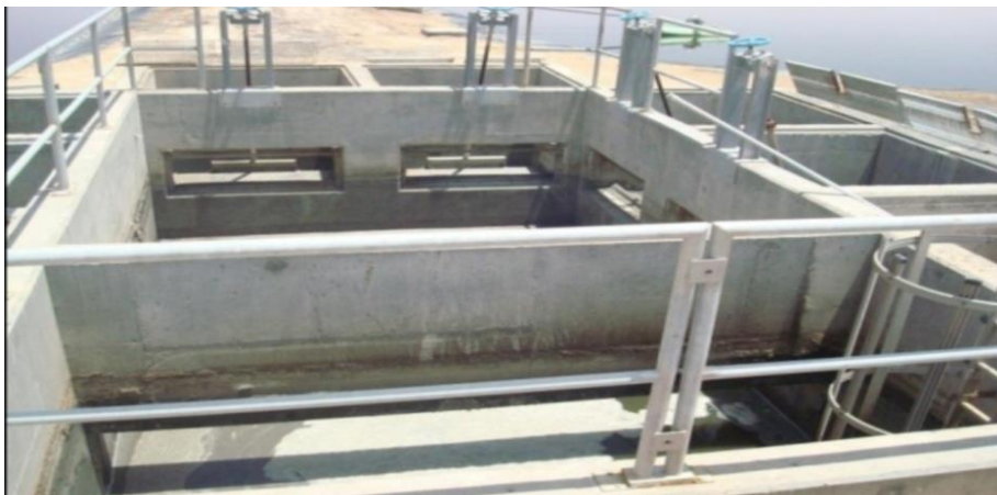
Fig (III. 8): Distributor to the aeration basin.
