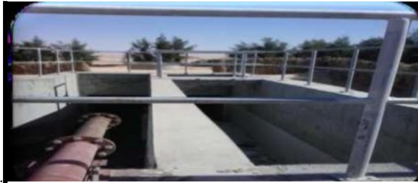
Fig (III. 10): Channels for transporting wastewater ( left ) and water drainage ( right ) in the Ouargla station [5].
