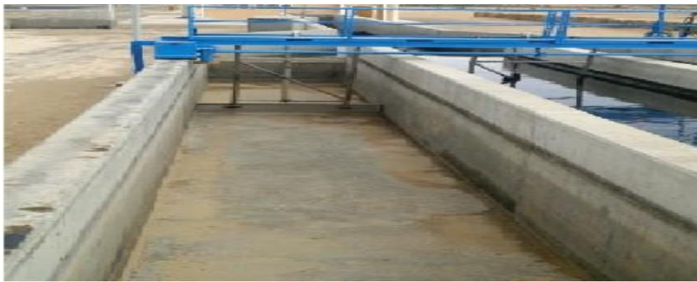
Fig (III. 7): Desanding in the Ouargla station.
