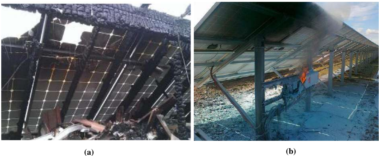
Fig. 1.6 Examples of fire occurred on: (a) Rooftop PV generator. (b) Junction box in a PV plant
