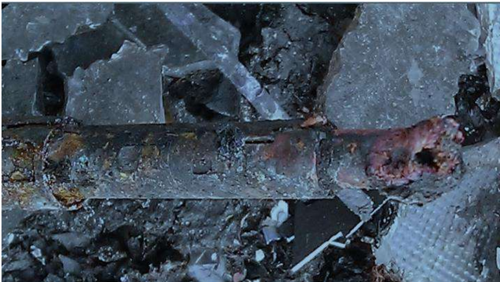
Fig. 1.4 DC cable melted due to electrical arcing in PV plant [29].
