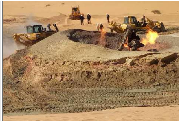
FigureI.4: MD244 Extinguishing Operation
