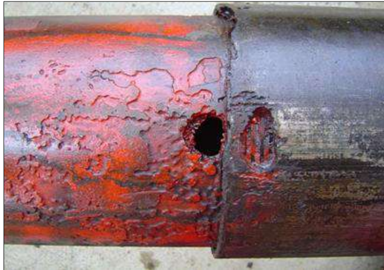
Figure I.12: Hole in the production tubing
