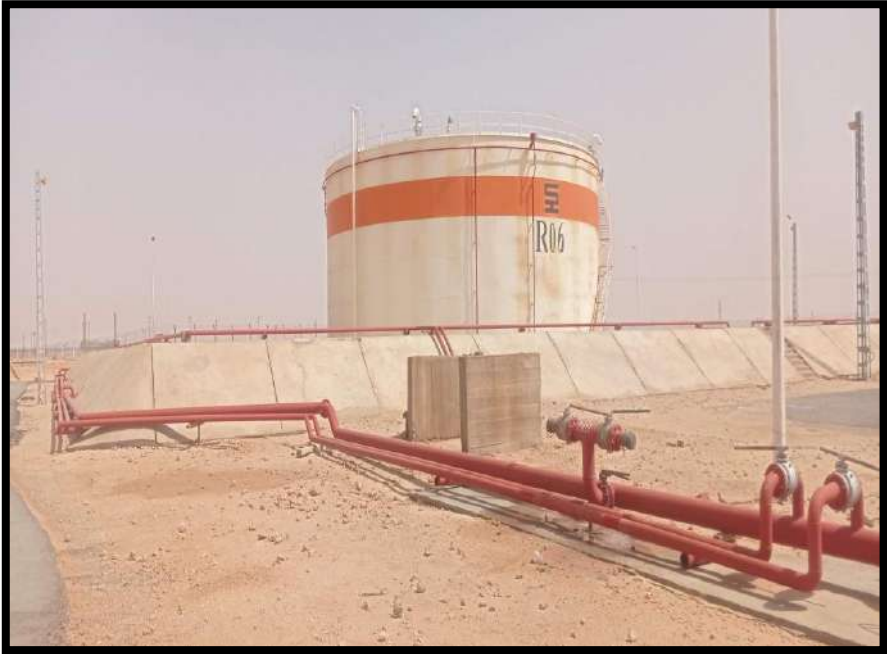
Figure II.5 Storage crude oil R06 and equipment of intervention cannon
