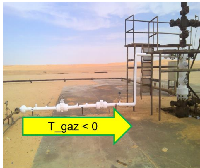
Figure II. 17: Example of Hydrates on Lift Gas Injection Line Downstream of Gas Lift Choke.
