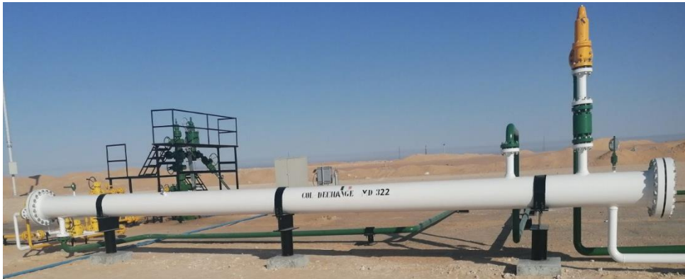
space between the platform and gas lift inlet line.
