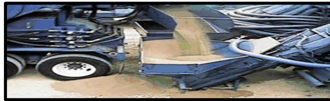
Figure I- 17 Frac sand being delivered from a Sand King to the hopper of a blender [2]
