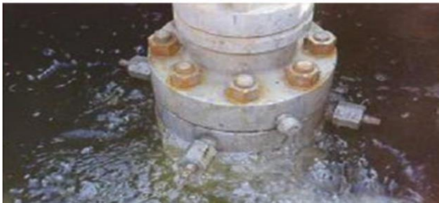
Figure II.8. Visual evidence of gas leakage; gas bubbles coming from the wellhead[2]
