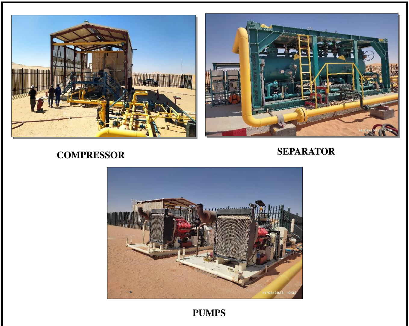
Figure III.3: Main equipment of the Boosting unit. [15]
