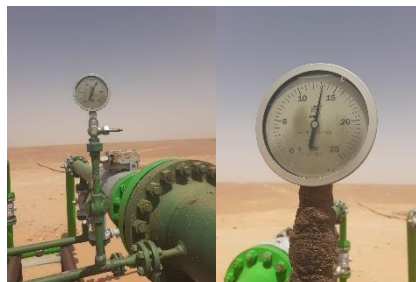
Figure II.9 : Pressure gauges mounted.
