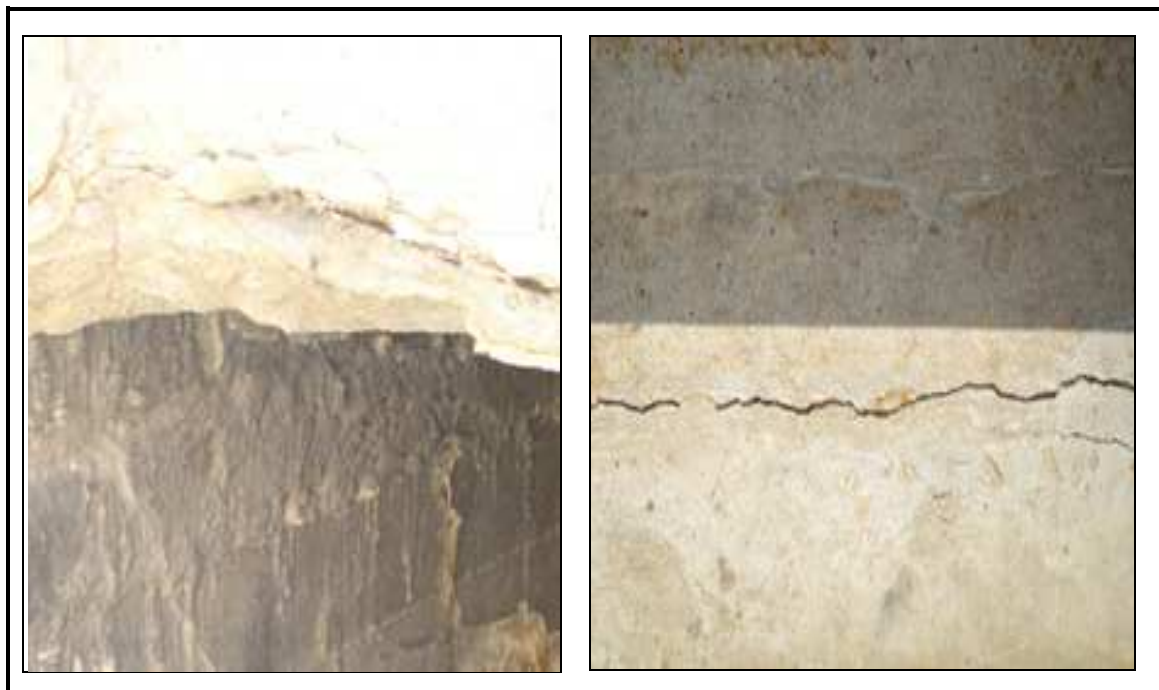
Photo (III, 6): Illustrations de fissuration horizontale -voile –
