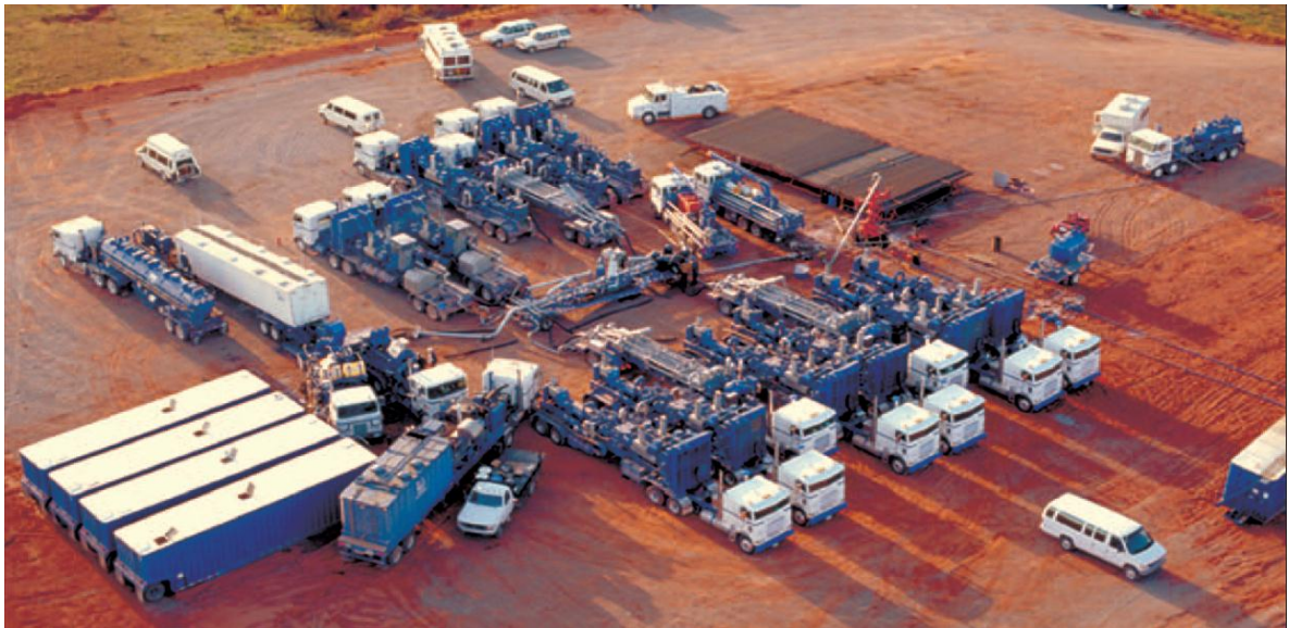
Figure II.2: Hydraulic Fracturing Equipment Onsite.
