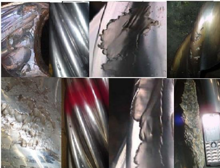
Figure (III.17): L'érosion de rotor.
