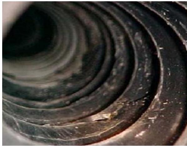
Figure (III.8): Délamination de stator.
