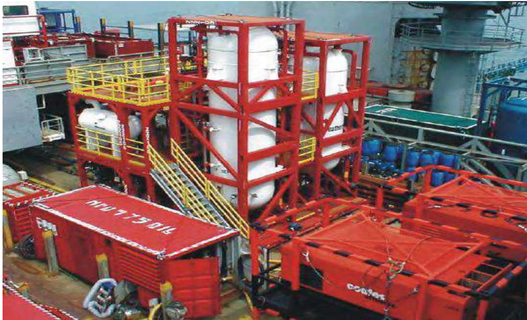
Figure 25 Multiphase Separation System for MPD 33
