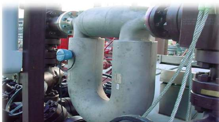
Figure I.10: Flow meter (A CMF 400M, Coriolis type).
