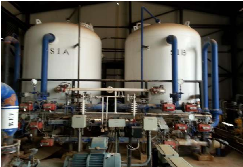
Fig.I.2: Filtres S01 A/B.
