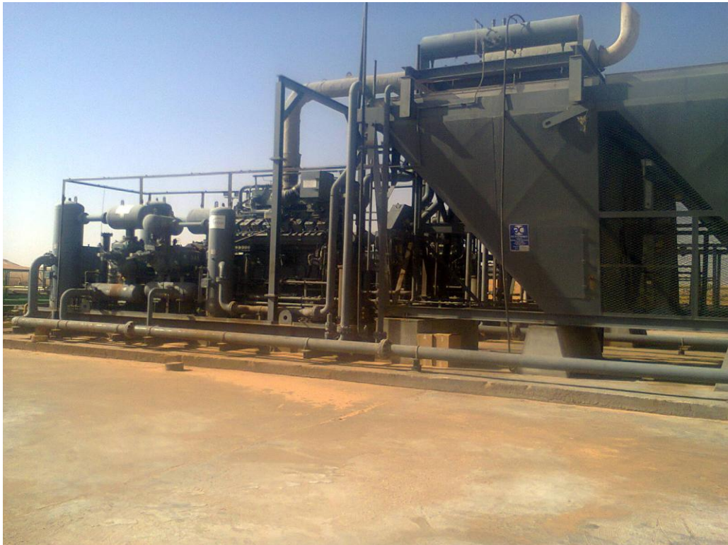
Fig.V.3 :Installation de compression
