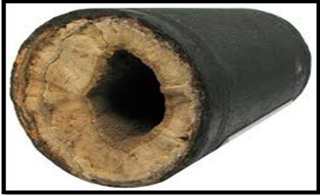
Figure: 1.5 DEPOT DE SULFATE DE CALCIUM (CASO4)
