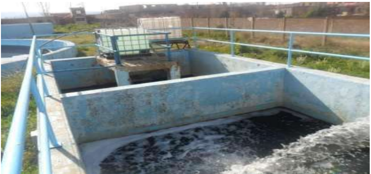
Figure IV.9 bassin de post chloration
