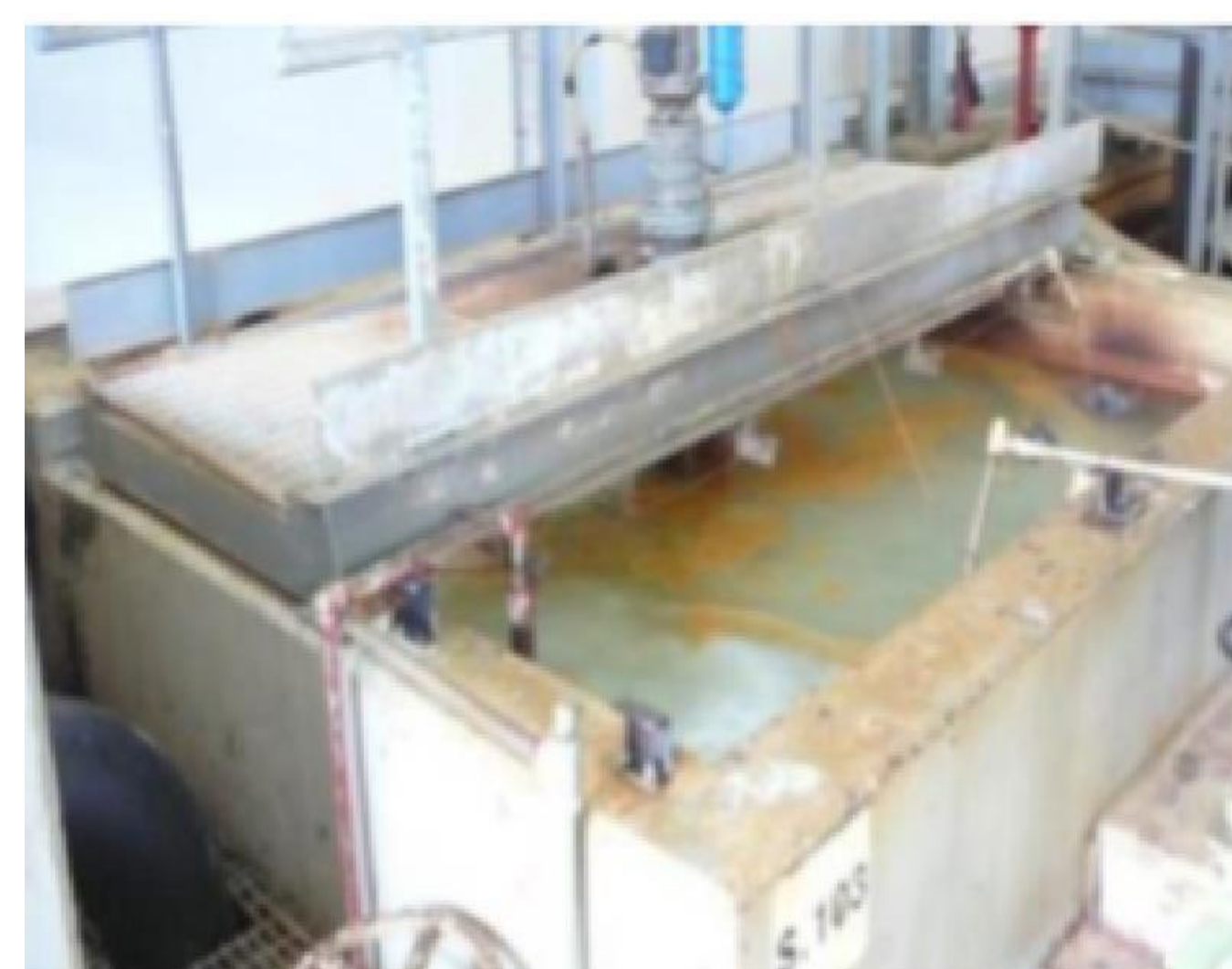
figure3: Photo de Cuve flocculation
