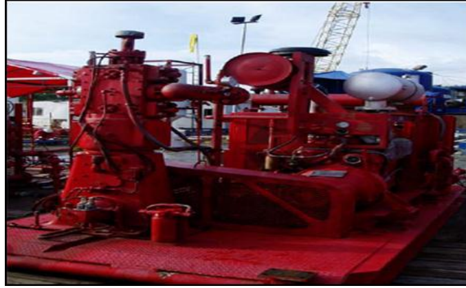
Fig. I.8. High pressure booster
