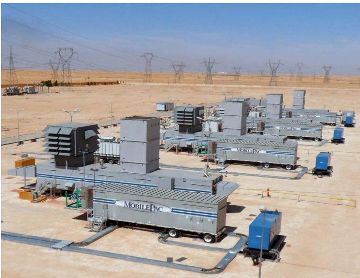
Figure 0-12: Centrale TG Mobile Hassi Messaoud HMO
