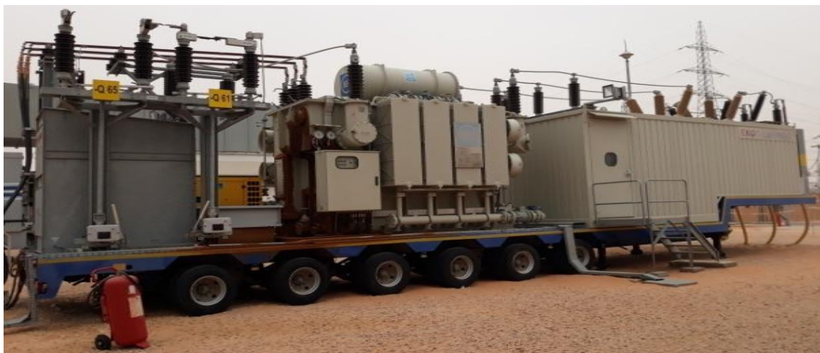
Figure 0-17: sous-station 11.5 kV -63 kV
