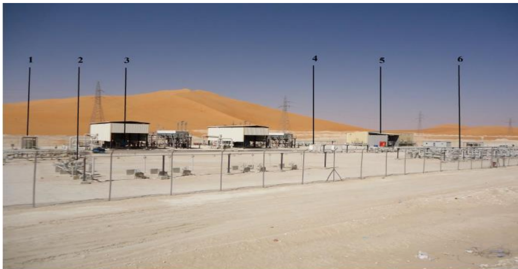
Figure I-10 : Installation de surface FGS
