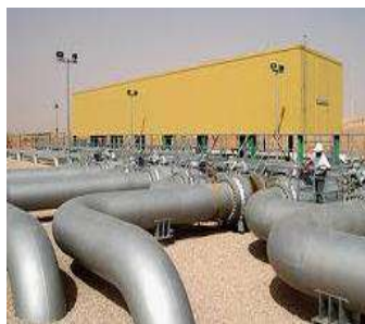
Figure II. 30: Station de pompage pétrolière[10]
