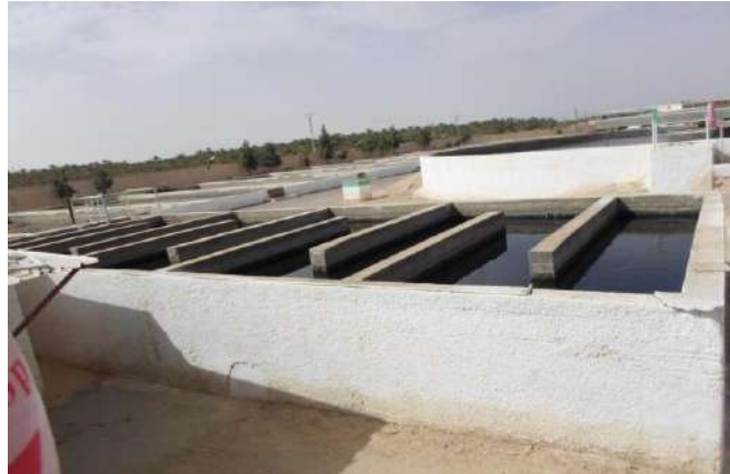
Figure III.11 Bassin de chloration
