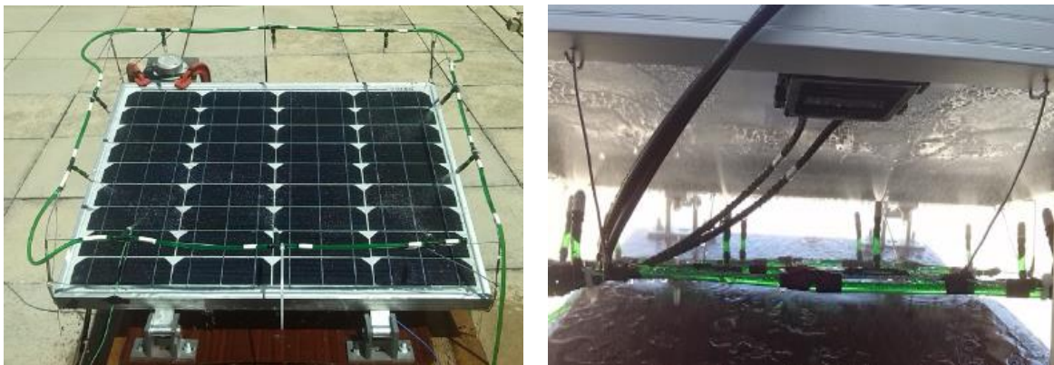
Figure 2-19 The front and backside cooling of PV panel by water spray system (Nižetić et al., 2016).
