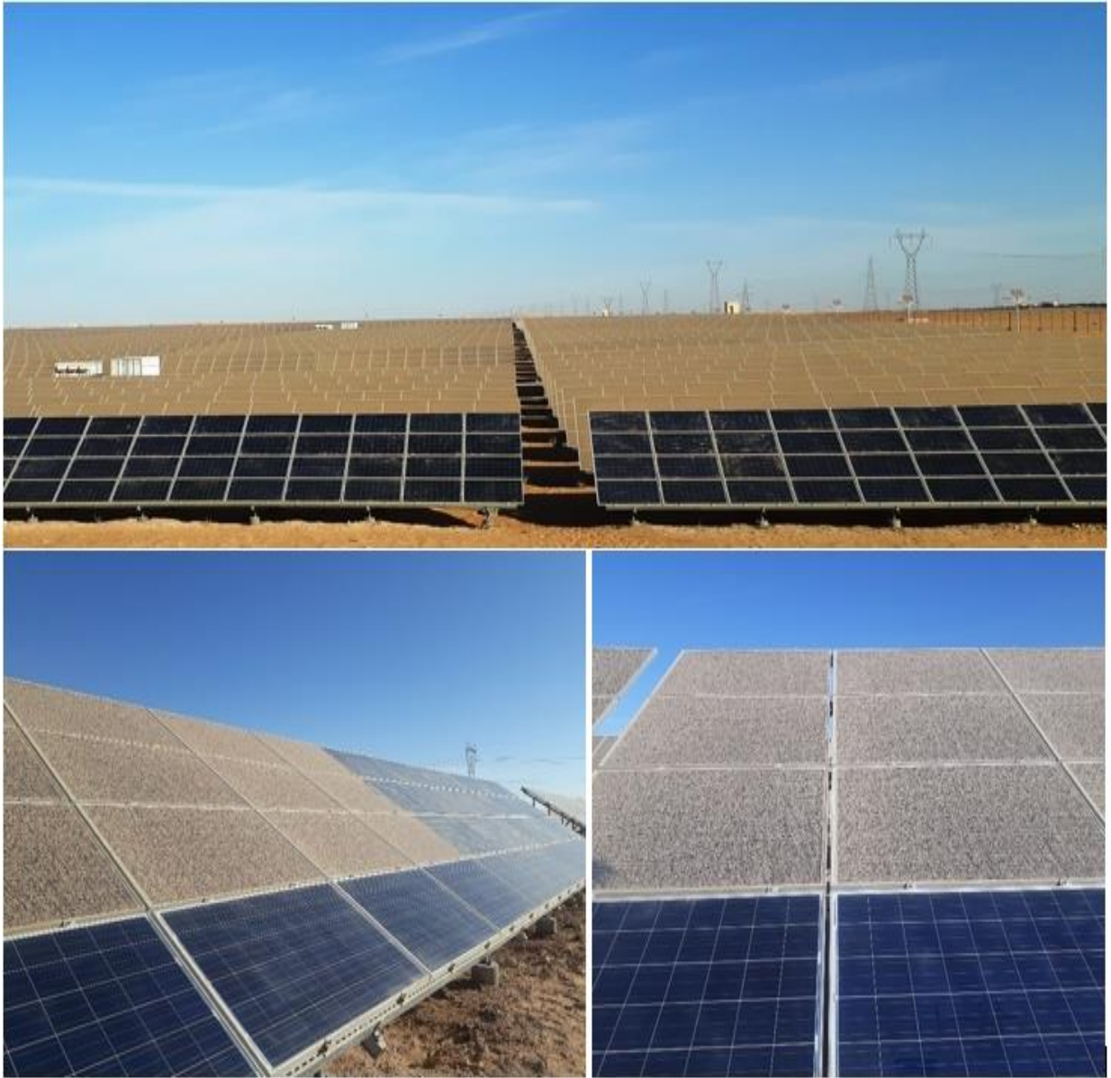
Figure 3-15 Photograph of accumulated dust on PV modules.
