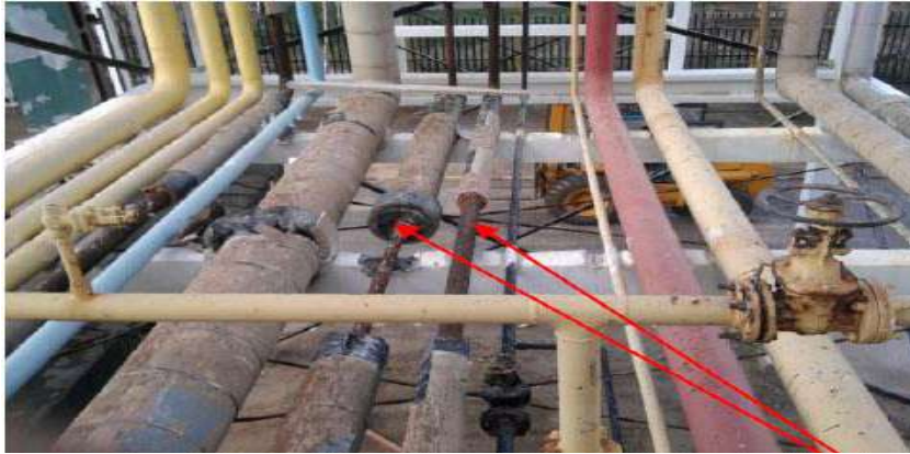
Fig1: Corrosion of lines in GL1K plant Skikda, Algeria 2004 ,before the blast occurred in January 20, 2004[5].
