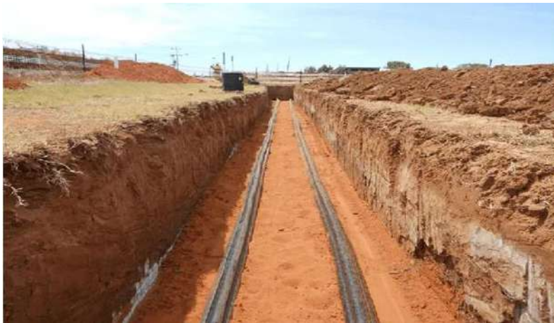
Figure I.1. Underground Power Cables.
