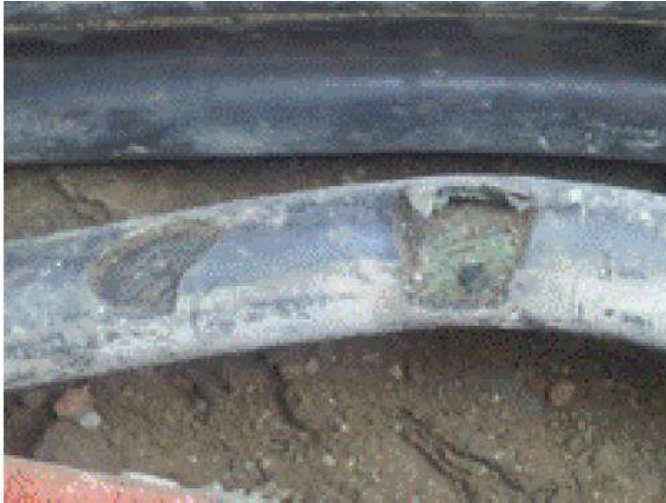
Figure I.25. Damaged 138 kV XLPE cable.[19]
