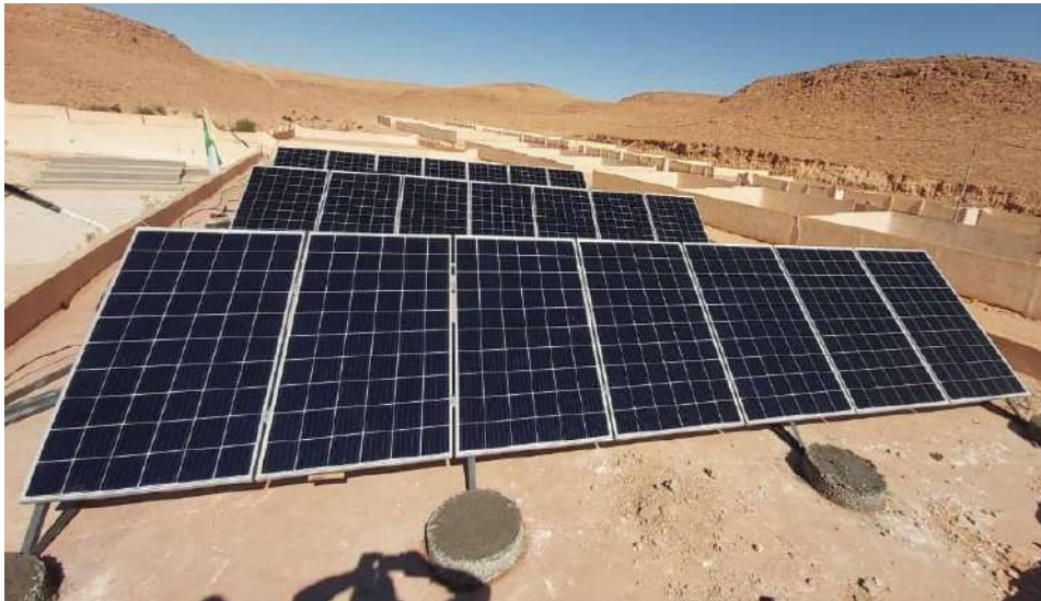
Figure III.8: Le champ photovoltaïque étudié
