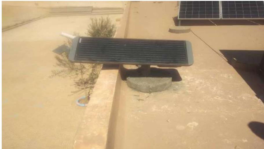
Figure III.7: Eclairage solaire extérieur -All in one
