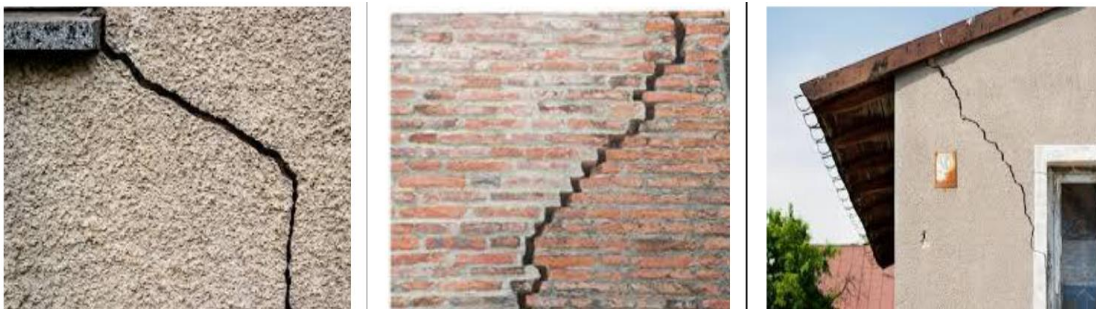
Figure (II.09) : Fissuration des murs.
