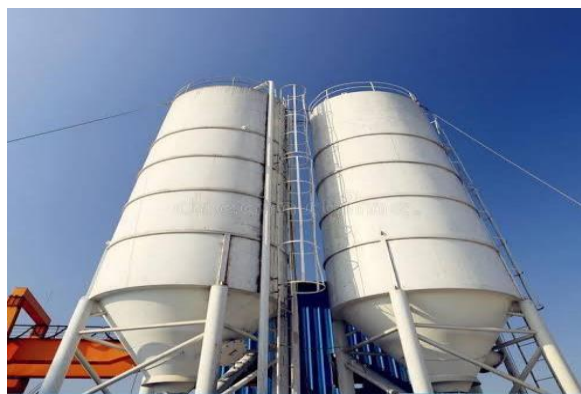
Figure I.28 : Silos de stockage
